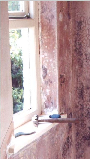
Wind blown rain caused the dampness problem in this lounge wall.
