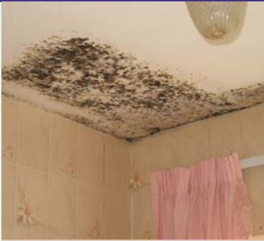
Mould grew on this bathroom ceiling because of missing insulation in the loft
