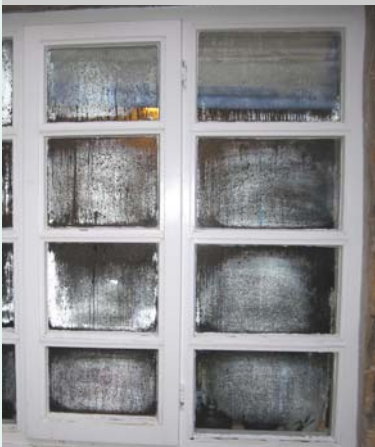
Persistent condensation affected every window in this house during the winter.
