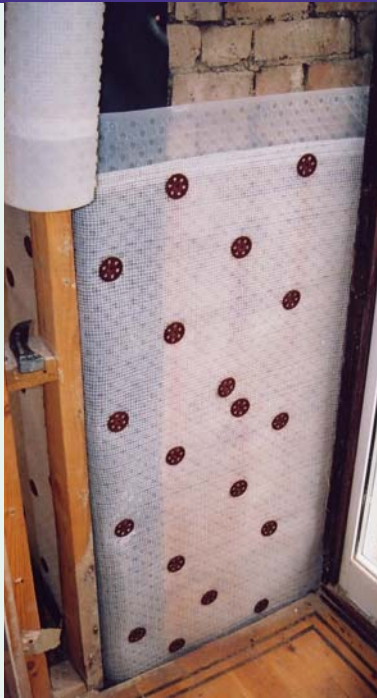
A ventilated damp proof barrier solved a persistent dampness problem for one of our clients
