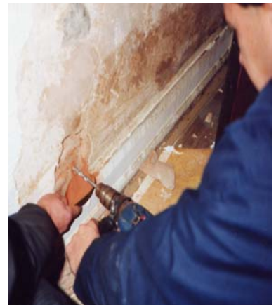
Sometimes taking samples of the wall is the only way to identify the damp.
