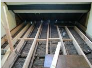
A surveyor failed to spot this loft floor was not strong enough. The repairs were very expensive.
