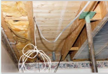
To stop the bedroom walls cracking, this floor had to be strengthened.
