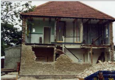
This wall collapsed because it was not properly connected to the rest of the house.
