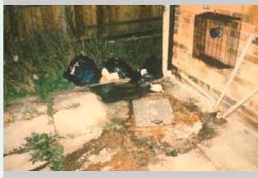
Unfortunately, some problems are only too obvious!
