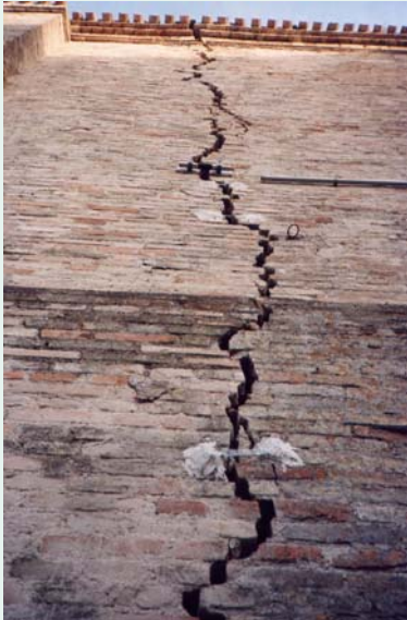
This crack in the side of an older building is being monitored to see if it gets bigger.
