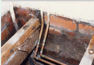
A plumbing leak resulted in wet rot to the end of these floor joists
