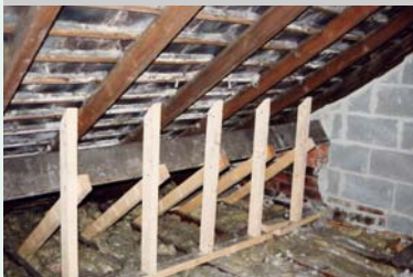
This weak roof structure was badly 'boded' by a builder who did not have a clue!
