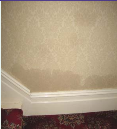
Damp areas to the base of a wall
