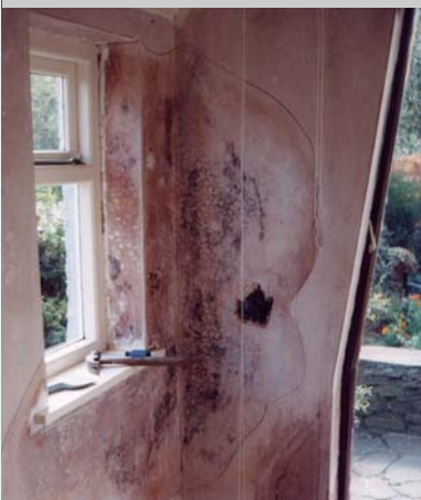
This problem was caused by rain water coming through cracks in the wall.
