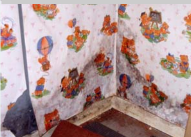
This dampness was caused by a problem in the floor rather than the wall.
