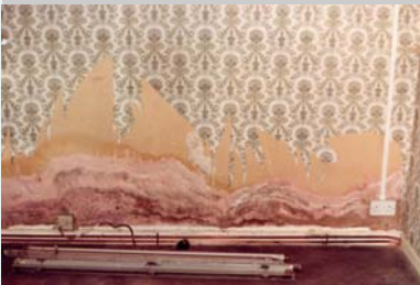
In the worst cases, dampness can cause 'tide marks' and affect the plaster
