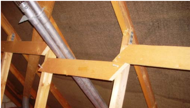
Hopefully, this building work is unauthorised!
