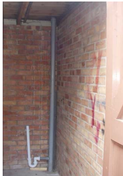
This shows a rain water pipe from a flat roof that connects into a separate surface water drain. No prizes for guessing what used to discharge into the new connection!
